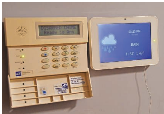
The IQ Panel 2 next to a legacy keypad. The only issue was the difficulty of hiding the antenna wire (right) when mounting to an exterior wall.
