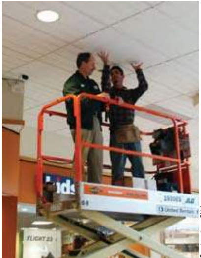
Tom Sutton (left), electrical inspector for Hamilton Township, and Ed Owens, an Arose electrician, conduct an above-ceiling inspection.
