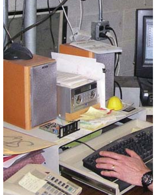
An electronic security system can be unreliable because of the application, hardware or installation. If the problems are a result of the application or hardware, campuses are usually better off replacing the system.
